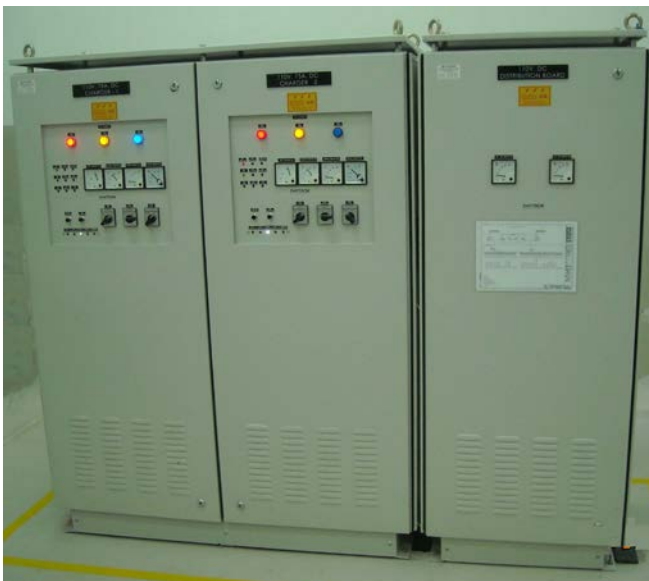
Dual Charger with DC Distribution Panel
